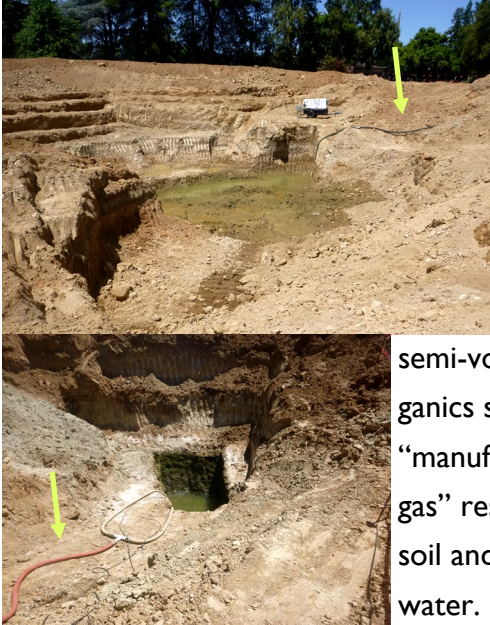
Site Mitigation on F Street—contaminated groundwater is pumped out, filtered and discharged to sanitary sewer (under permit).
