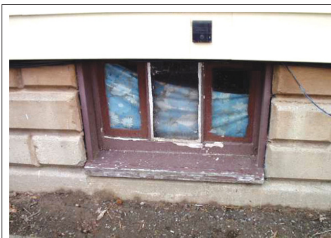
FIGURE 6.3 An area of bare soil beneath a window with deteriorated paint.
