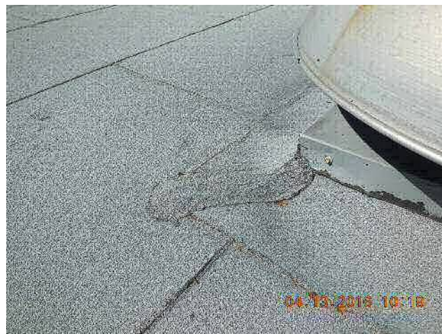
Visible Roof Discoloration at Vent
