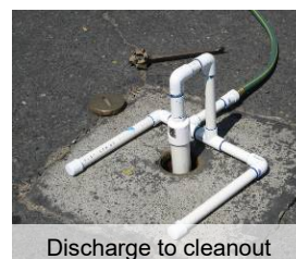
Discharge to cleanout
